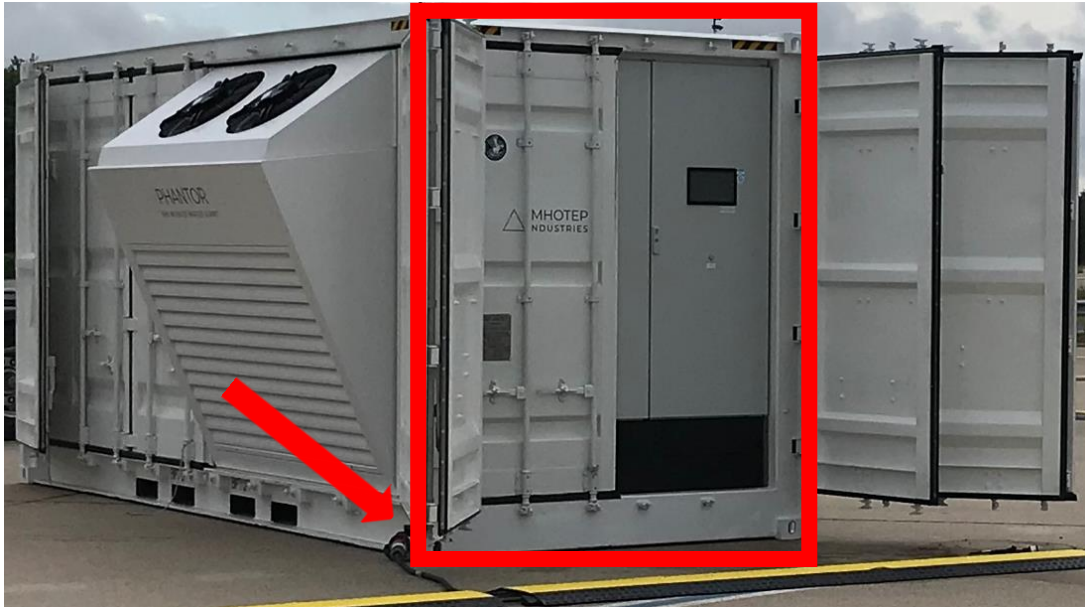
Figure 3: Electrical junction box at the front with cable entry (arrow)
