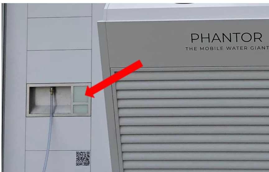
Figure 17: Water kiosk with RFID card reader (arrow)
