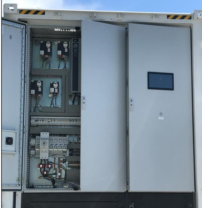
Figure 5: Electrical junction box interior view
