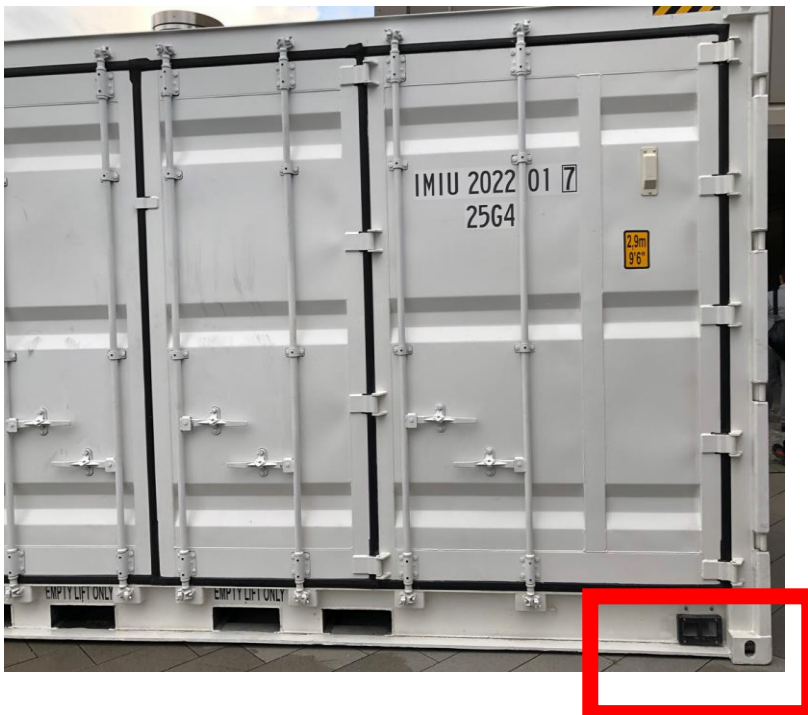
Figure 4: Cable entries below
