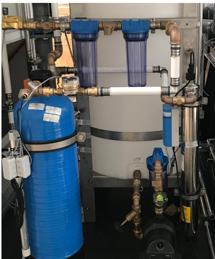
Figure 15: Water treatment (filter, UV disinfection, deacidification/mineralization)
